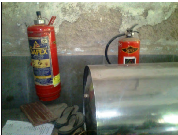
Picture: Fire extinguishers obstructed with equipments
