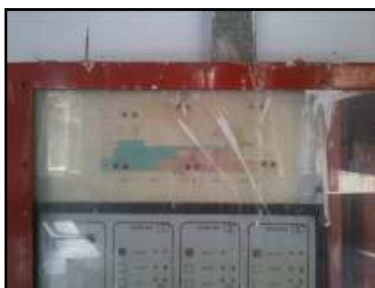
Fig 4.1 Fire Panel- First Floor
